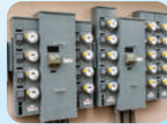
Energy Management System
