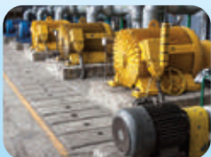
Pump Station Management
