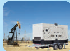
Outdoor Generator Monitoring
